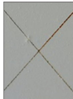
Fig. 1 — Teslan 2-coat system, 8.5 total mils.
