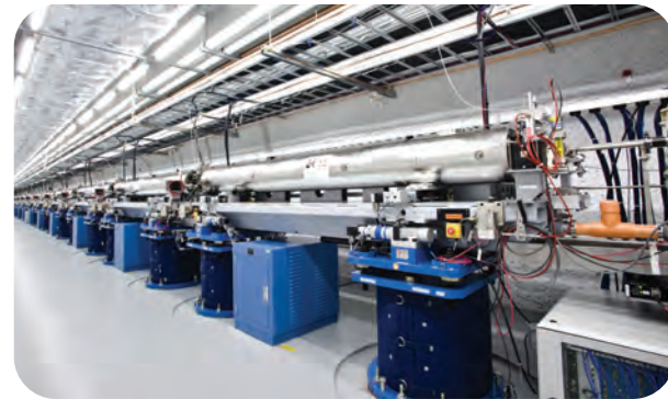
The Undulator Hall of SLAC Lab's Linac Coherent Light Source, which "wiggles" electrons to generate high-power coherent x-rays crucial to studying superconductivity.
